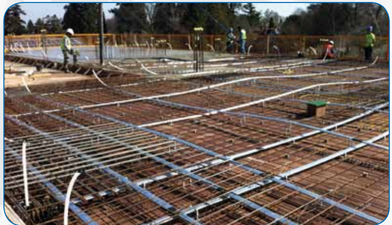
A typical post-tensioning installation.
