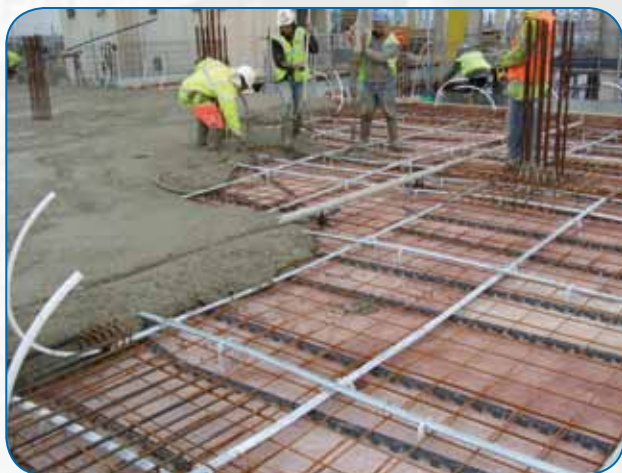
The Middlehaven CIAC project in Middlesbrough. For more information see [2]. Photo: supplied by CCL.
